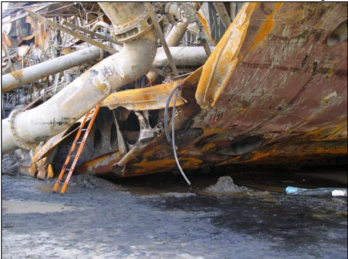
Starboard side hull collapse near lower sea chests
