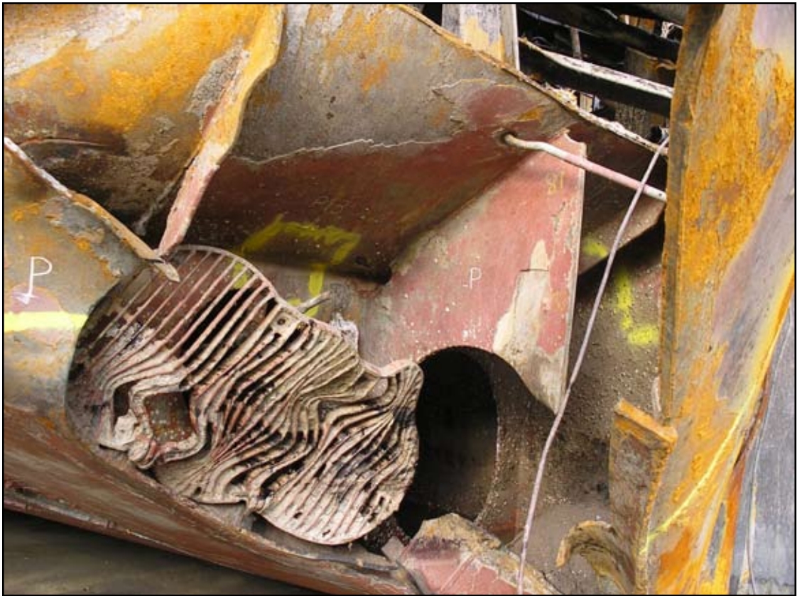
Localised plate buckling - port sea chest
